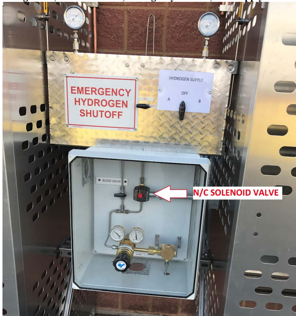
Typical Outdoor Control Features Regulator, Solenoid Valve, Emergency Shutoff, Gas Supply Valve
